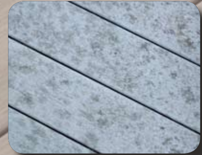
Mold on composite decking
